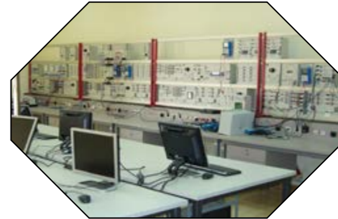
Electrical Power Systems Laboratory.
